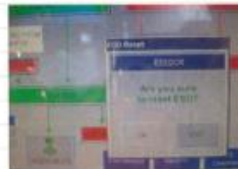
Fig33: Test ESD from HMI to ESDV
