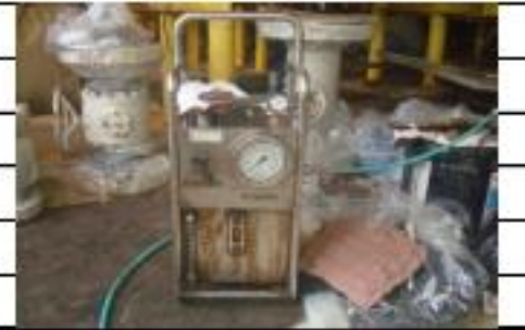
Fig3 : Flushing pump for Olivals-VF
