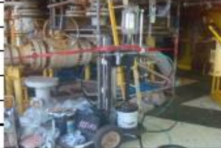
Fig5 : Lubricant / Sealant pump
